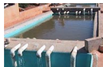
Washing water purification system
